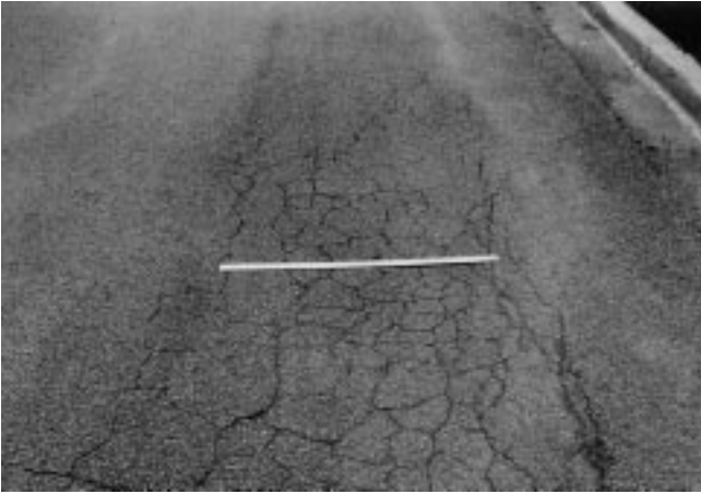
FIG. X1.2 Medium-Severity Alligator Cracking
