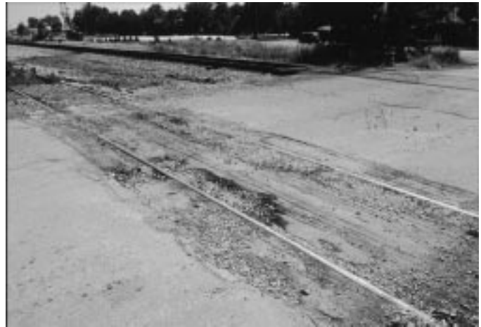
FIG. X1.40 High-Severity Railroad Crossing
