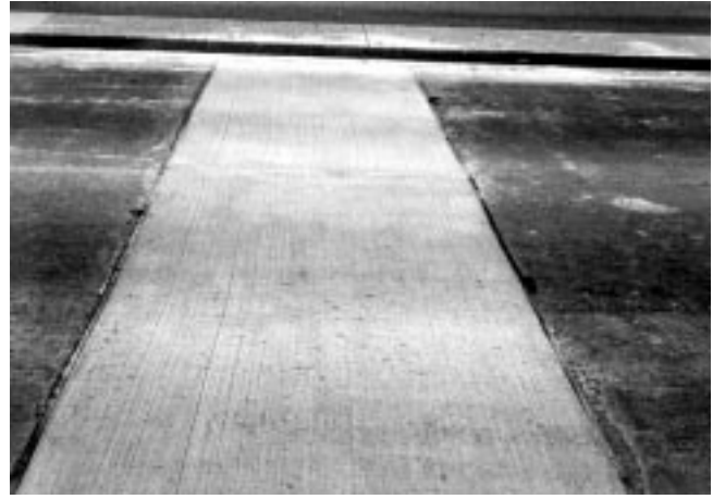
FIG. X2.25 Low-Severity Patching, Large and Utility Cuts
