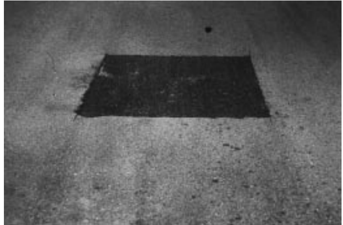
FIG. X1.31 Low-Severity Patching and Utility Cut Patching
