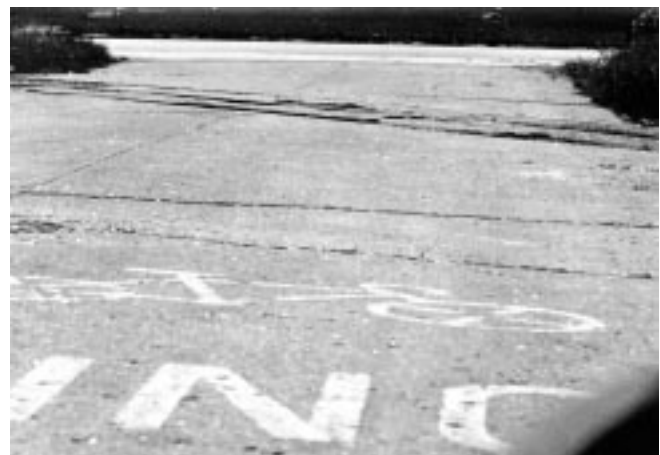
FIG. X2.39 Medium-Severity Railroad Crossing
