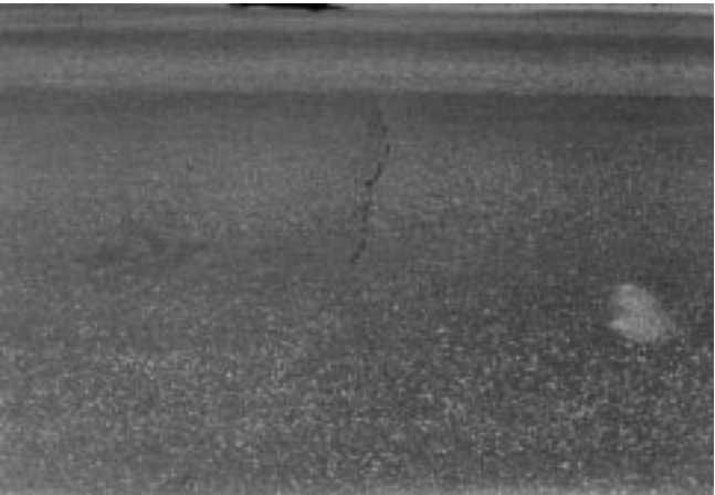
FIG. X1.28 Low-Severity Longitudinal and Transverse Cracking
