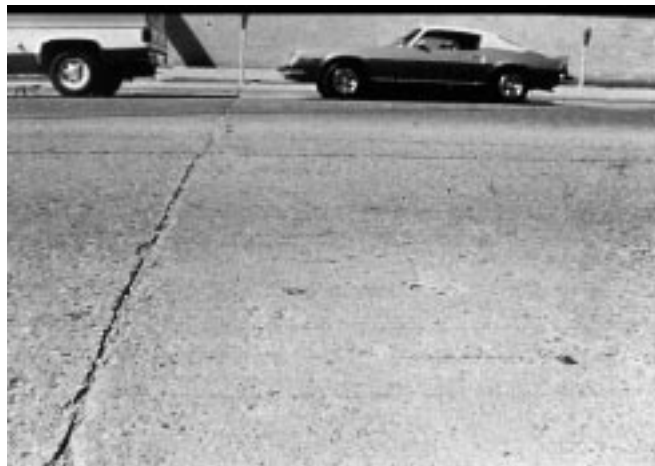
FIG. X2.48 Low-Severity Spalling, Joint
