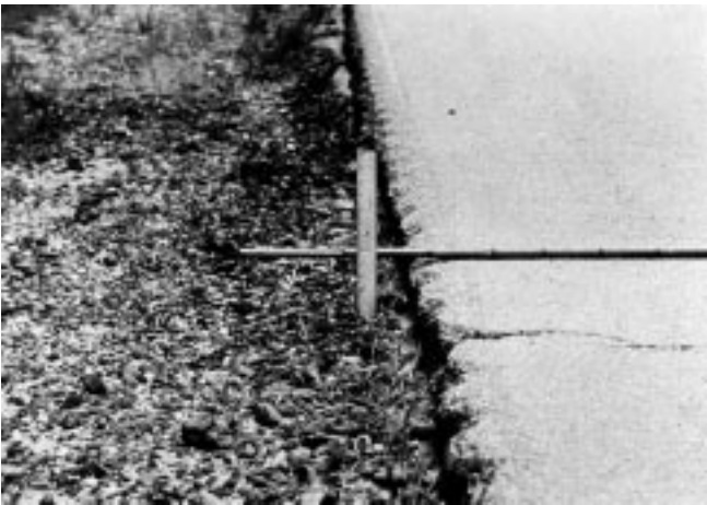
FIG. X1.27 High-Severity Lane/Shoulder Drop-Off
