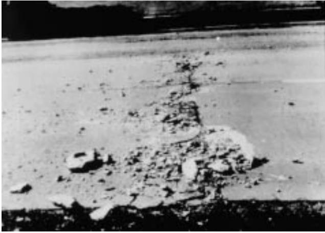
FIG. X2.2 Medium Severity Blowup/Buckling
