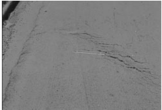
FIG. X1.48 Medium-Severity Slippage Cracking
