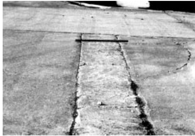
FIG. X2.26 Medium-Severity Patching, Large and Utility Cuts
