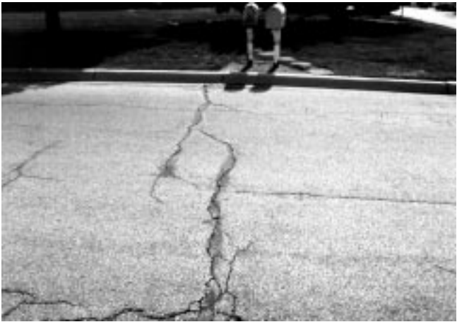
FIG. X1.8 Medium-Severity Block Cracking
