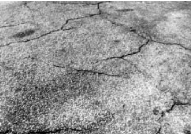
FIG. X1.9 High-Severity Block Cracking
