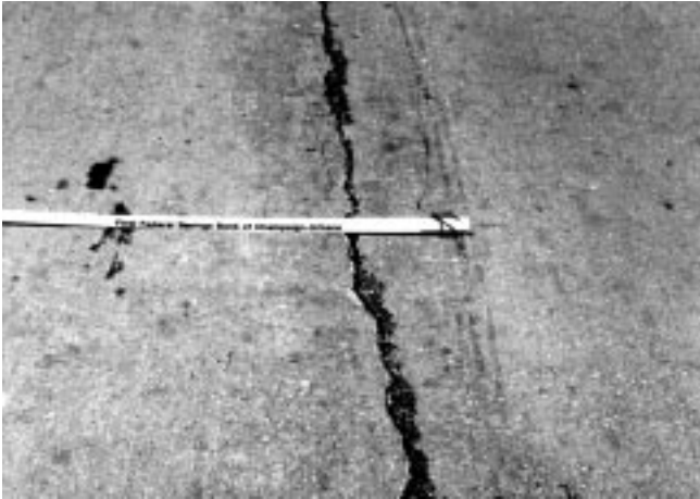
FIG. X2.23 Medium-Severity Linear Cracking
