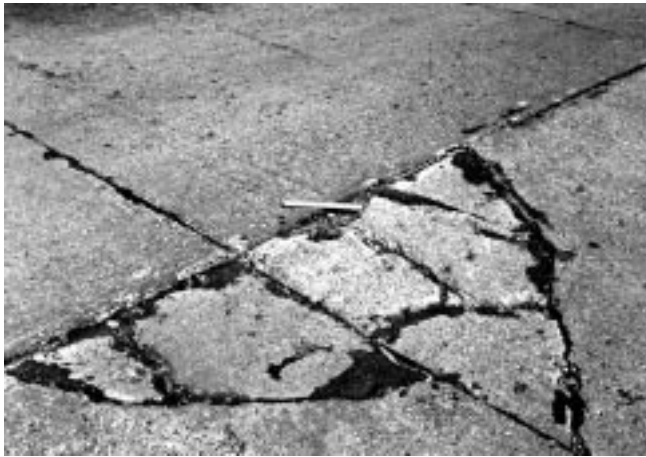
FIG. X2.6 High-Severity Corner Break
