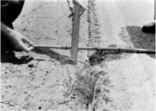
FIG. X1.26 Medium-Severity Lane/Shoulder Drop-Off
