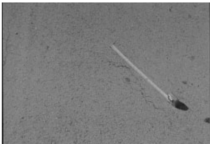
FIG. X1.47 Low-Severity Slippage Cracking
