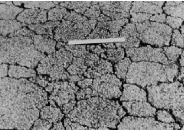
FIG. X1.3 High-Severity Alligator Cracking
