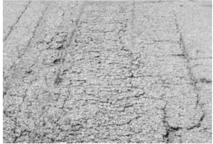
FIG. X1.52 Medium-Severity Weathering and Raveling
