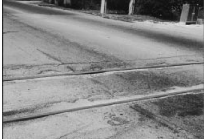
FIG. X1.39 Medium-Severity Railroad Crossing
