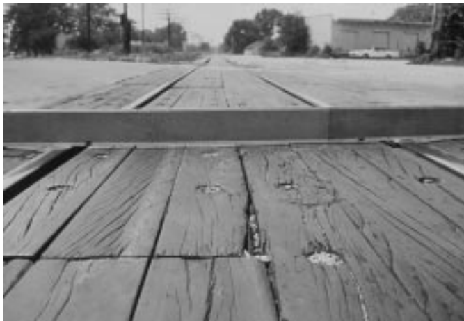
FIG. X1.38 Low-Severity Railroad Crossing
