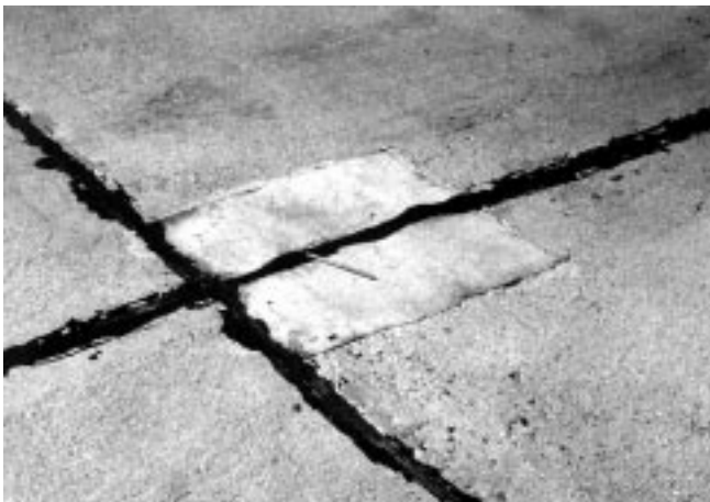
FIG. X2.28 Low-Severity Patching, Small
