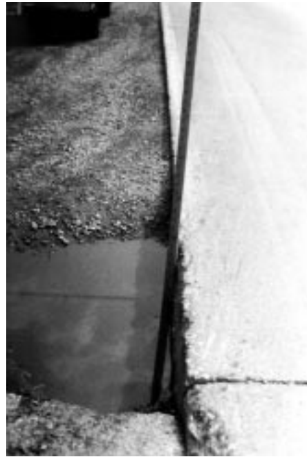
FIG. X2.21 High-Severity Lane/Shoulder Drop-Off
