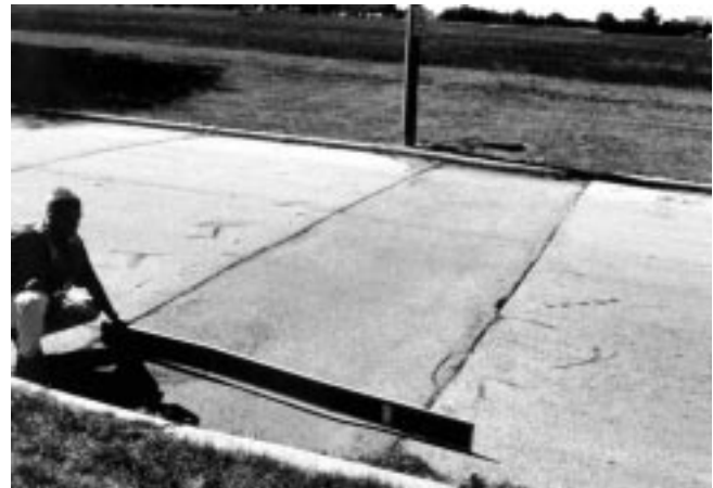
FIG. X1.32 Medium-Severity Patching and Utility Cut Patching
