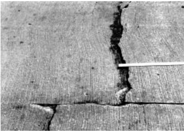
FIG. X2.24 High-Severity Linear Cracking
