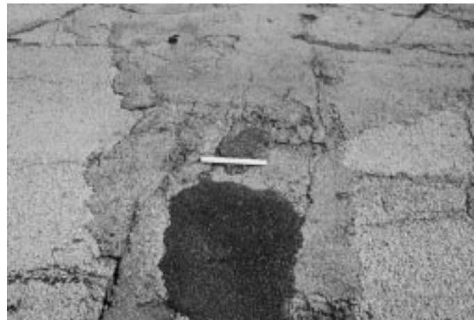
FIG. X1.33 High-Severity Patching and Utility Cut Patching
