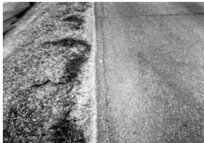
FIG. X1.19 Low-Severity Edge Cracking
