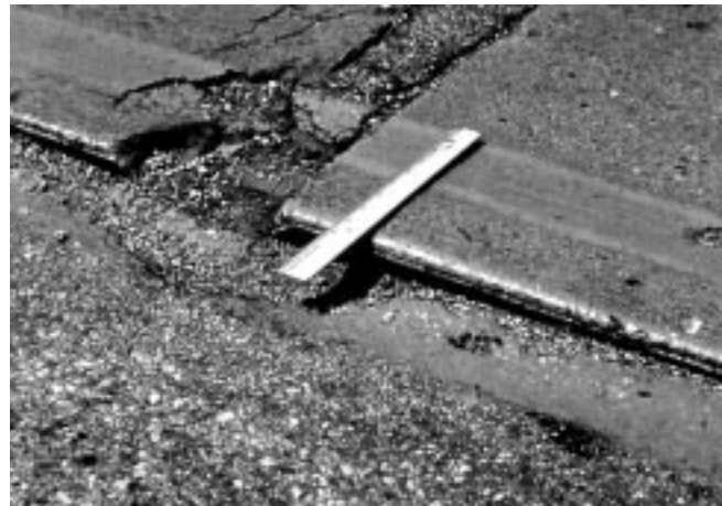
FIG. X2.19 Low-Severity Lane/Shoulder Drop-Off
