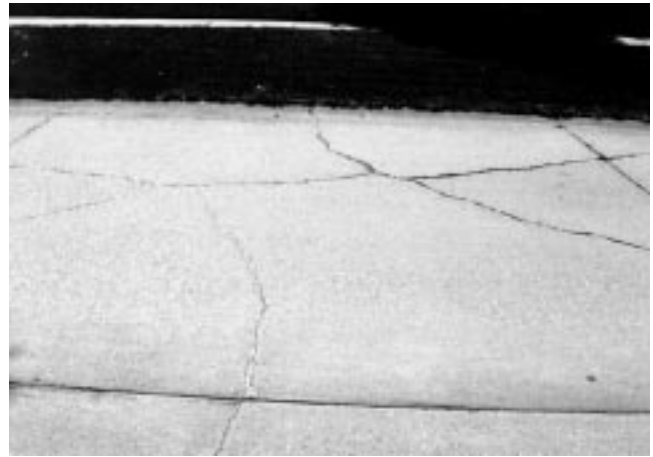
FIG. X2.8 Medium-Severity Divided Slab
