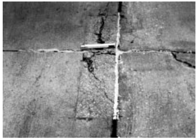
FIG. X2.30 High-Severity Patching, Small
