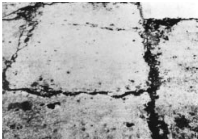
FIG. X2.27 High-Severity Patching, Large and Utility Cuts
