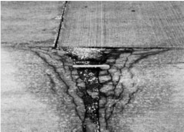
FIG. X2.11 Medium-Severity Durability Cracking
