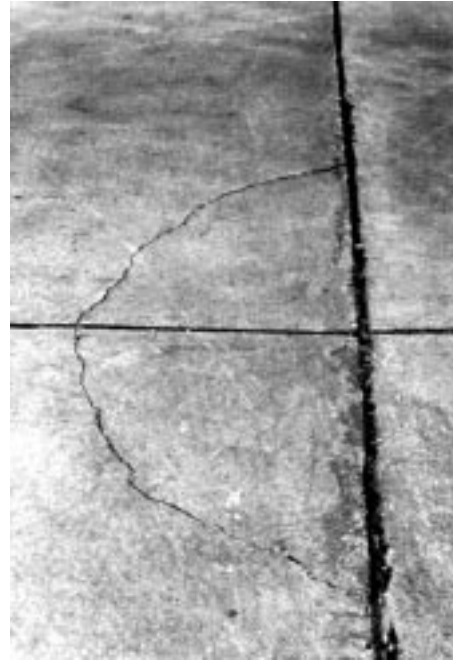
FIG. X2.4 Low-Severity Corner Break
