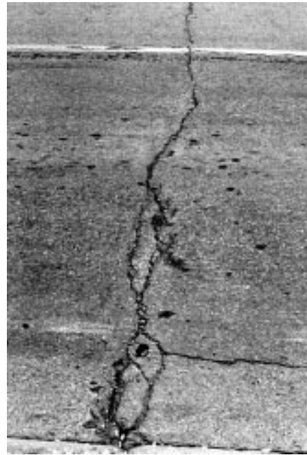
FIG. X1.23 Medium-Severity Joint Reflection Cracking
