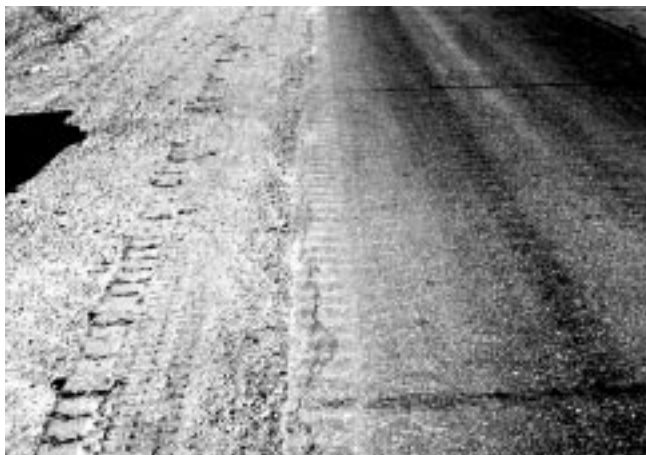
FIG. X1.22 Low-Severity Joint Reflection Cracking
