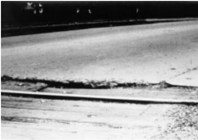
FIG. X2.40 High-Severity Railroad Crossing
