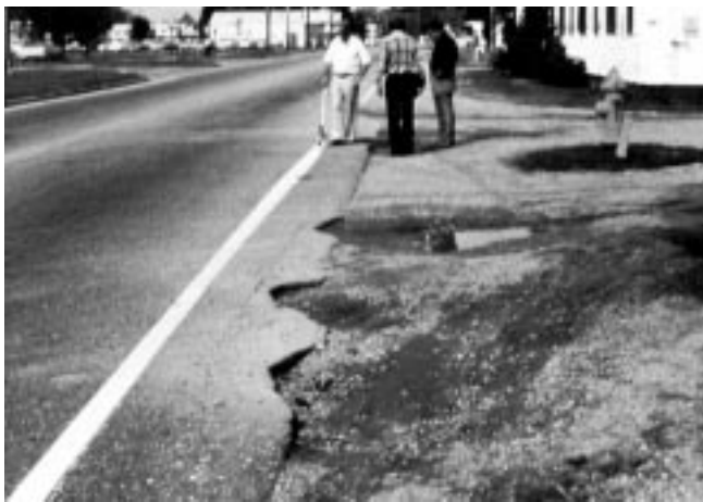
FIG. X1.21 High-Severity Edge Cracking
