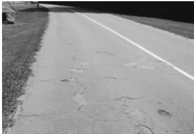
FIG. X1.53 High-Severity Weathering and Raveling
