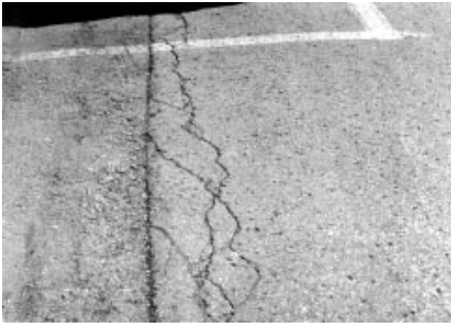
FIG. X1.20 Medium-Severity Edge Cracking
