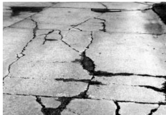
FIG. X2.9 High-Severity Divided Slab
