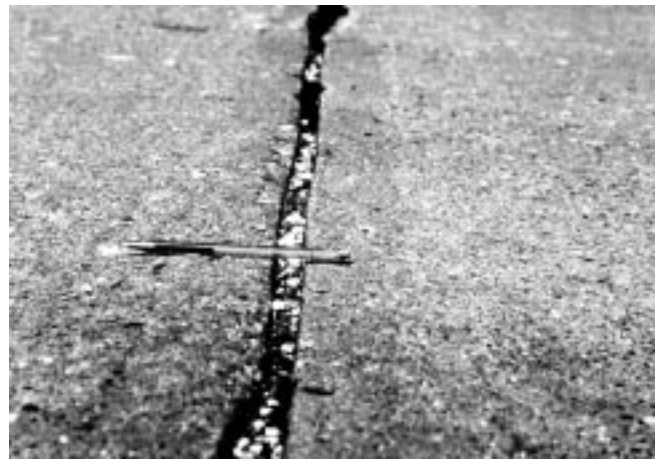
FIG. X2.18 High-Severity Joint Seal Damage
