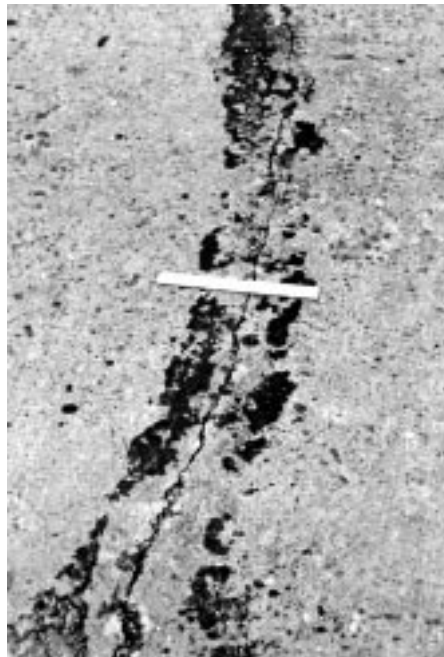
FIG. X2.22 Low-Severity Linear Cracking
