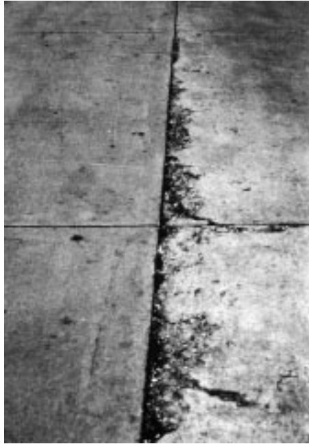
FIG. X2.49 Medium-Severity Spalling, Joint
