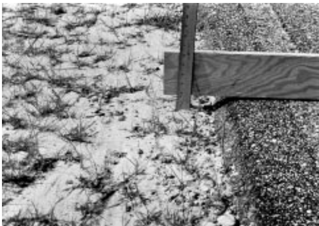
FIG. X1.25 Low-Severity Lane/Shoulder Drop-Off
