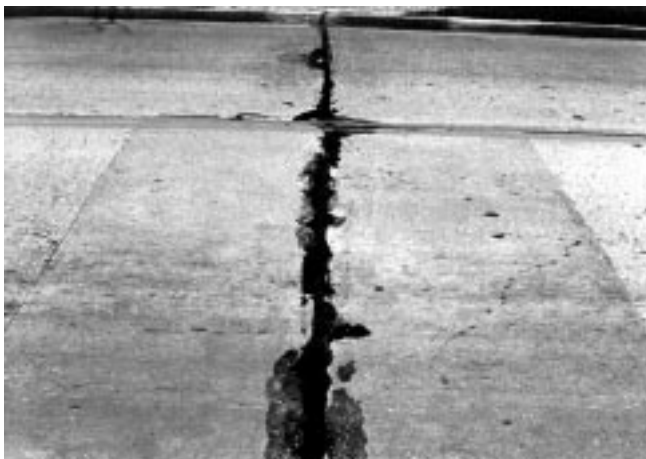
FIG. X2.16 Low-Severity Joint Seal Damage
