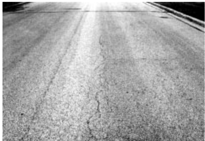
FIG. X1.1 Low-Severity Alligator Cracking
