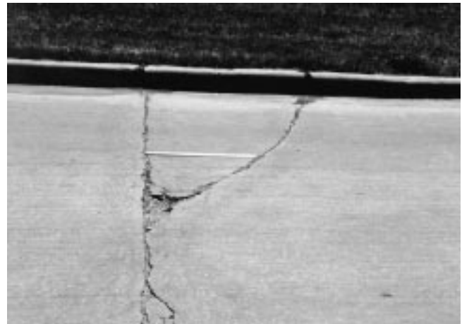
FIG. X2.5 Medium-Severity Corner Break
