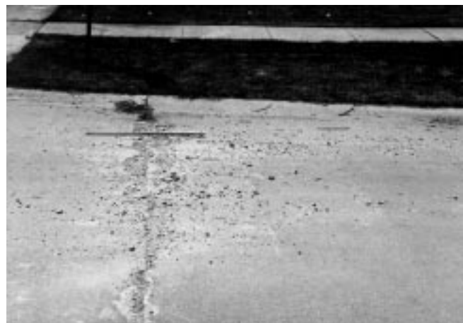
FIG. X2.1 Low Severity Blowup/Buckling
