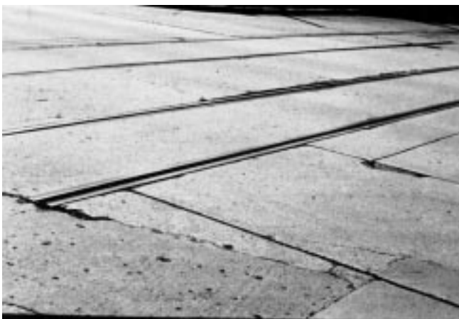
FIG. X2.38 Low-Severity Railroad Crossing
