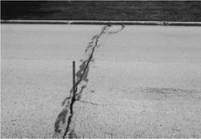
FIG. X1.29 Medium-Severity Longitudinal and Transverse Cracking
