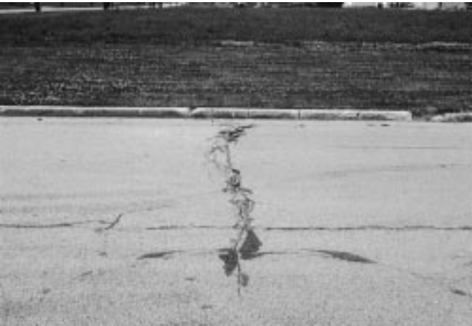
FIG. X1.30 High-Severity Longitudinal and Transverse Cracking
