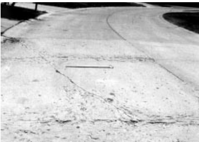
FIG. X2.12 High-Severity Durability Cracking
