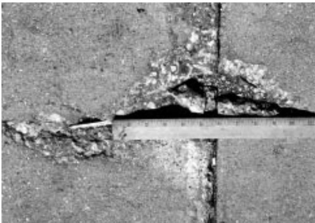
FIG. X2.46 Medium-Severity Spalling, Corner
